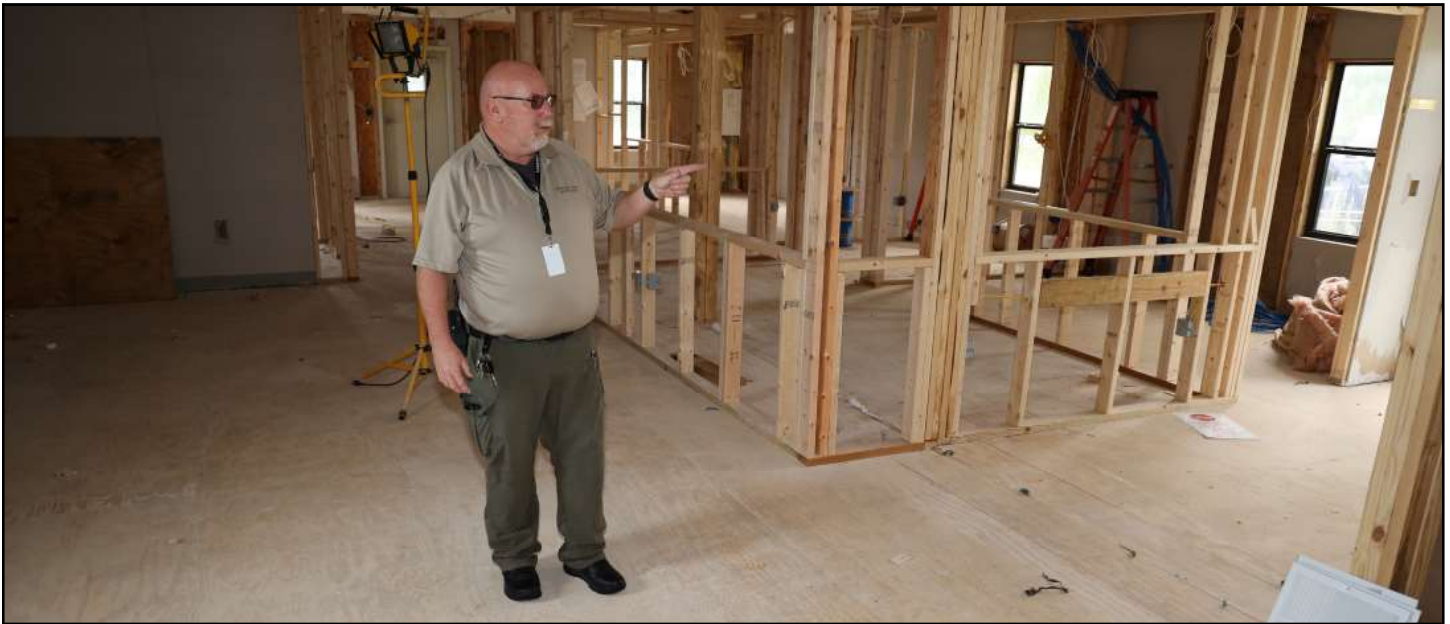
MAINTENANCE UNIT SUPERVISOR CHARLES WILLIAMS INSPECTS THE RENOVATIONS THAT WILL BECOME THE NEW VISITATION BUILDING.
